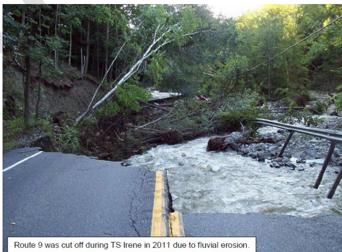
Route 9 was cut off during TS Irene in 2011 due to fluvial erosion.
